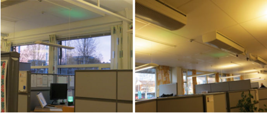
Fig. 6.6 The reflection of the “NEAT Lamp” on the ceiling represents an intersection between interaction design and architecture
